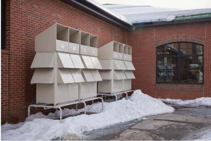
VRF Heat Pump System
